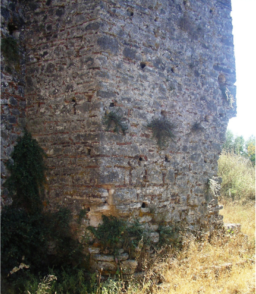
Fig. 226. Nea Kerassounda, Castle of Rogoi. Section of masonry in the N cross wall.
